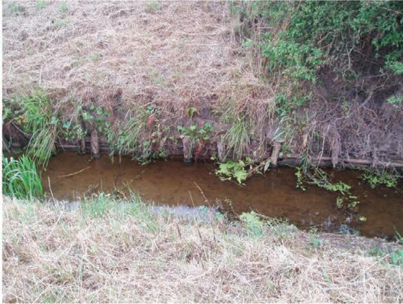
Plate 3. An example of the wooden revetment in Black Dyke, undertaken by the drainage board
